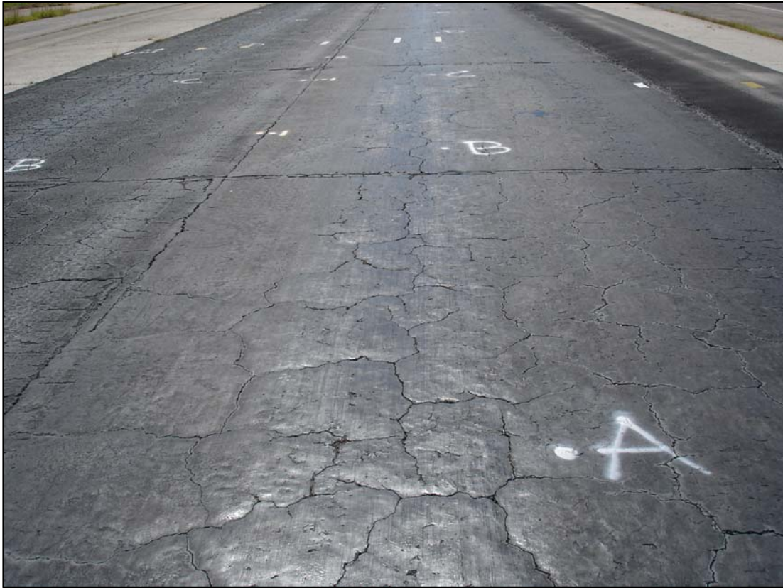
Figure 3. Skid Pad 2A.
